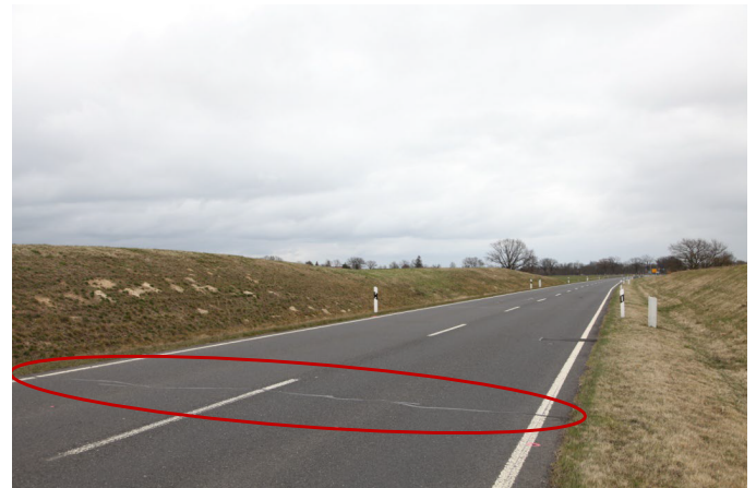
Fig. 9. Discontinuities (cracks) in the asphalt pavement structure
