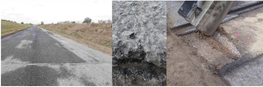
Fig. 11. Visible cracks on top of the asphalt base course and excavation
