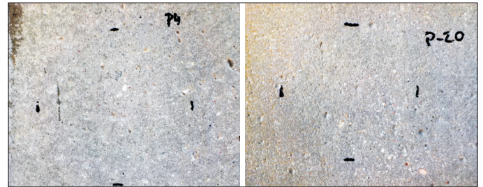
Fig. 9. View of concrete surface at measurement points nos. 4 and 20
