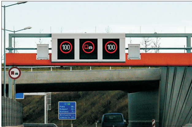
Fig. 2. Example of a pictogram VMS; on its both sides there are signs with continuous drawing [7]
