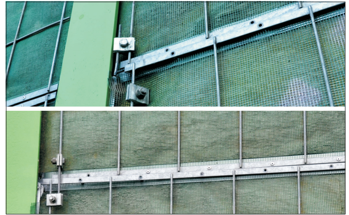
Fig. 3. Sheared/torn out rivets fastening the steel mesh to horizontal profiles
