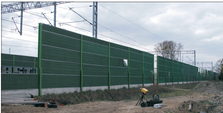
Fig. 5. The first investigated section: from the left (direction of incoming trains) a span with removed panels, the tested span no. 6-7 with accelerometers (installed on the top of the columns and the panel), visible interferometric radar for displacement measurements
