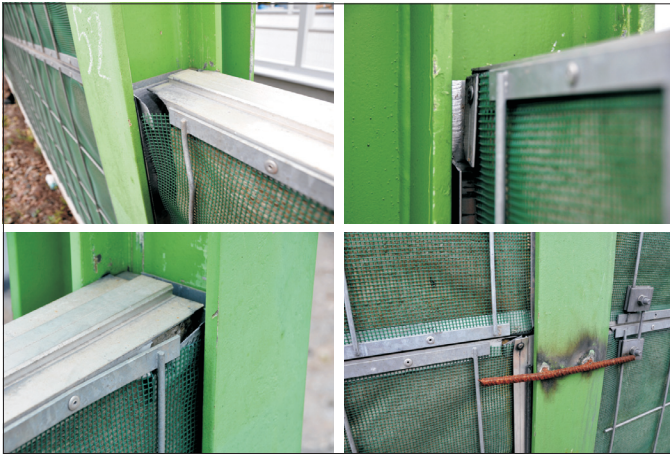
Fig. 2. Transverse and longitudinal cracks in the corners of horizontal and vertical profiles of the panel frame, in the vicinity of rivets
