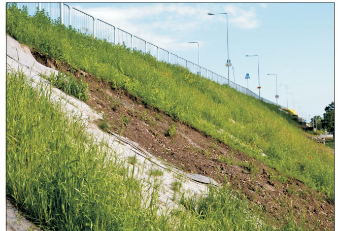
Fig. 6. The rainfall-induced local slope failure on section protected with anti-erosion mats (June 2019)
