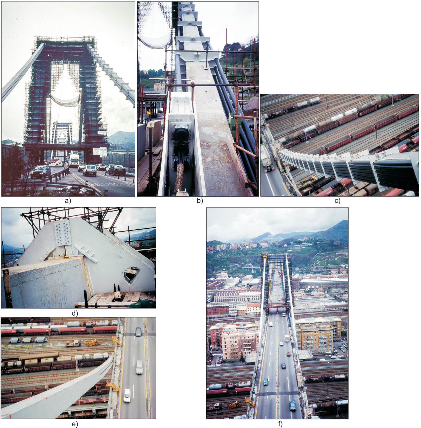
Fig. 6. a) Support No. 11 with strengthened north-eastern concreted cable, b) Strengthening of the concreted cable with long external tendons - view from the deck, c) The north-western concreted cable after strengthening - view from the top of pylon No. 11, d) Steel cap on pylon No. 11, e) The south-western concreted cable before strengthening - view from the top of pylon No. 11, f) View from the top of pylon No. 11 to pylon No. 10 with scaffolding (photos by J. Rymysz; 04.1993)
