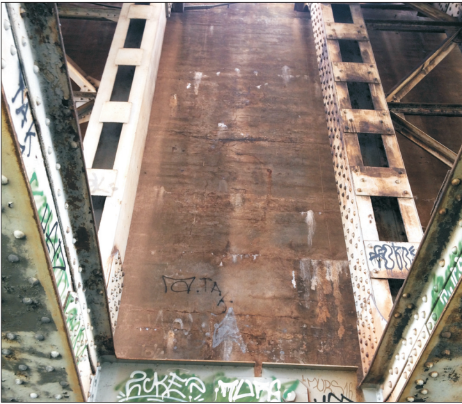
Fig. 1. Noticeable defects of a concrete resistance wall caused by simultaneously appearing failure phenomena including alkali-aggregate reactions
