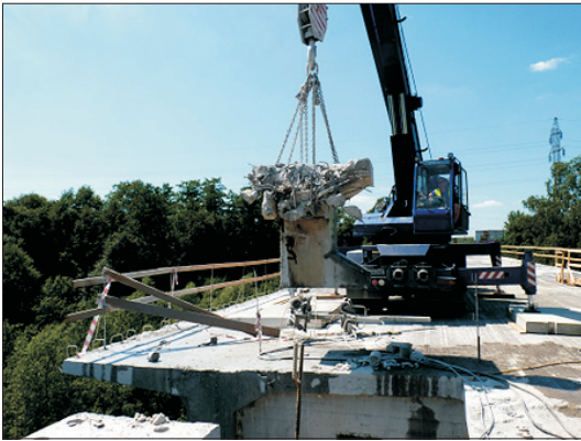
Fig. 12. Removing of the degraded central parts of the bridge in the place of joint
