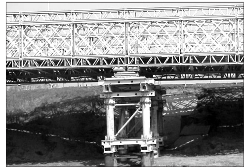
Fig. 3. Variant II of a construction, the DMS-65 bridge reinforced with a spatial overlay
