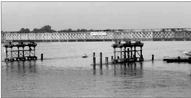
Fig. 2. Variant I of a construction, the basic configuration of the DMS-65 bridge
