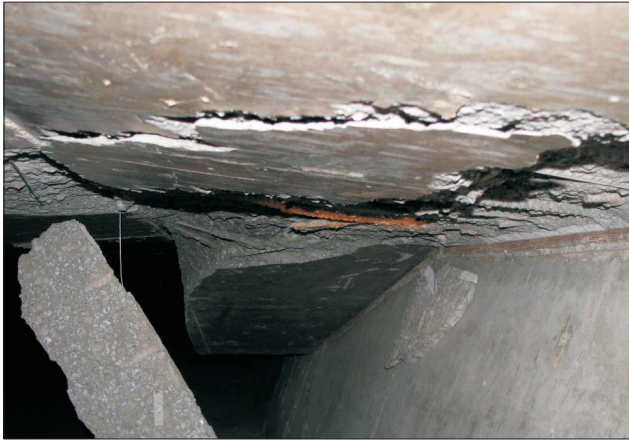
Fig. 3. View of the top slab of the box cross-section directly after failure
