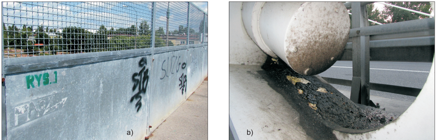
Fig. 5. Dirt: a) graffiti on railings, b) leakage of a substance that protects a cable against corrosion (own photos)
