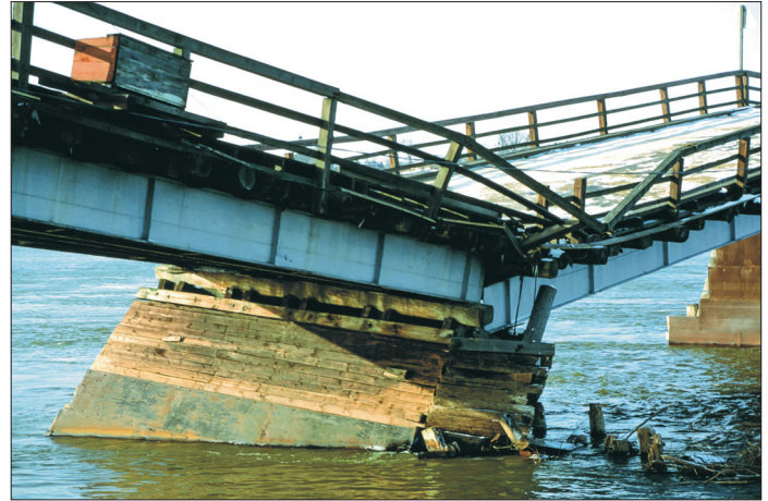
Fig. 3. Destruction of one pier and two spans caused by the ice drift in spring 1993, photo: Marek Mistewicz [7]
