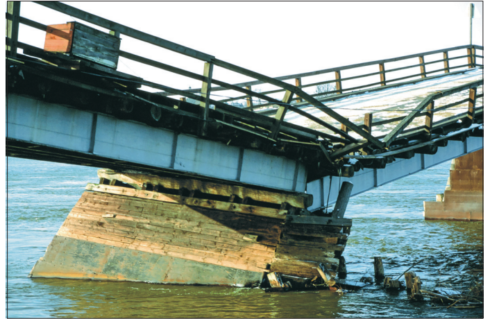
Fig. 3. Destruction of one pier and two spans caused by the ice drift in spring 1993, photo: Marek Mistewicz [7]
