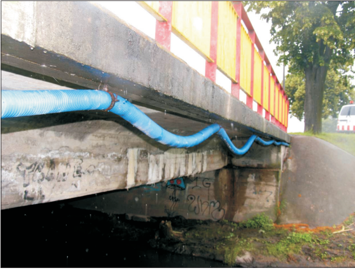
Fig. 3. Bridge side view – visible leakages of calcium carbonate on the side of the slab and on the abutment wall
