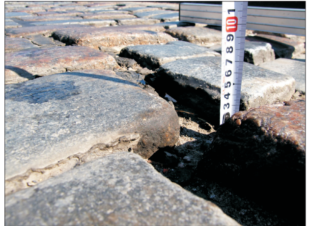
Fig. 6. Lacks of filling in joints up to 4 cm
