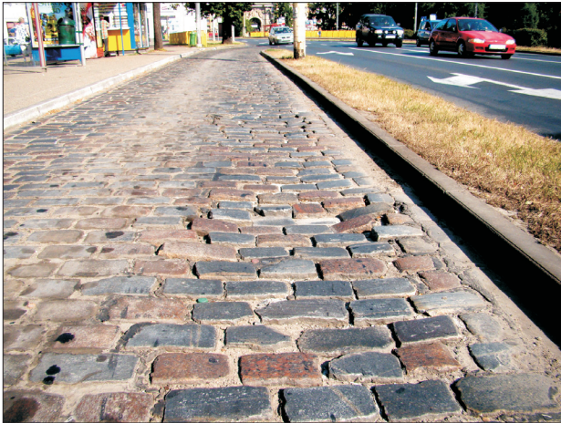
Fig. 5. Pavement laid on subgrade made of debris and unclassified subgrade
