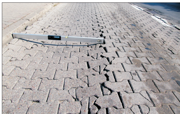
Fig. 1. Examples of failure to fill in joints and broken concrete blocks
