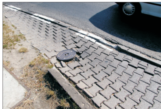
Fig. 2. Examples of protruding manholes, broken or lacking curbs, which make impossible the application of measuring devices
