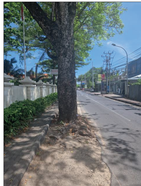
Fig. 10. Example of a tree planted close to the edge of the road, damaging the road pavement and the sidewalk – Bali (Indonesia)
